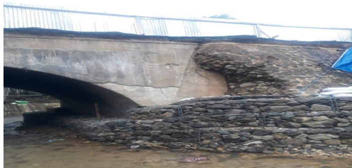
Gambar 2. Keruntuhan Elemen Abutmen Akibat Longsor
